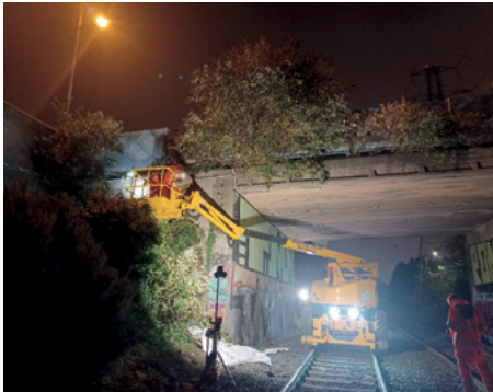
T3 possession: At night this is the most common and safest system
